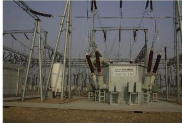
Fig. 7. A few of the 220 kV/0.8 kA superconducting fault current limiters after installation at Sjhigezhuang substation in Tianjin
